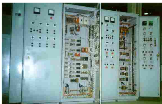
The modular board for gas transferring unit control. Ordered by NPO ISKRA, Perm.
