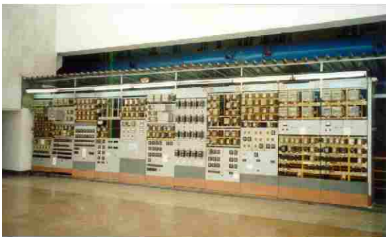
The relay switchboard at a distribution substation
