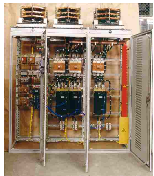
The control case for a pumping station
